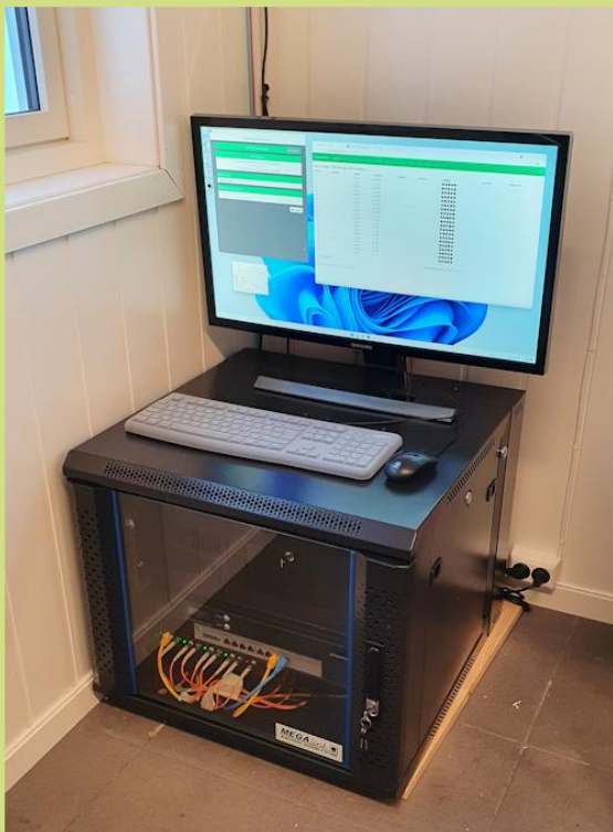
Compact unit with server and UPS for continuous use.
